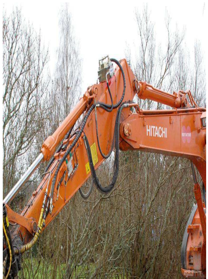
PRESSURE COMPENSATOR INSTALLED TO A PRESSURE PORT OF A MAIN HYDRAULIC PUMP
